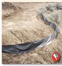
Silt fence is installed backwards; posts should be on downhill side.
